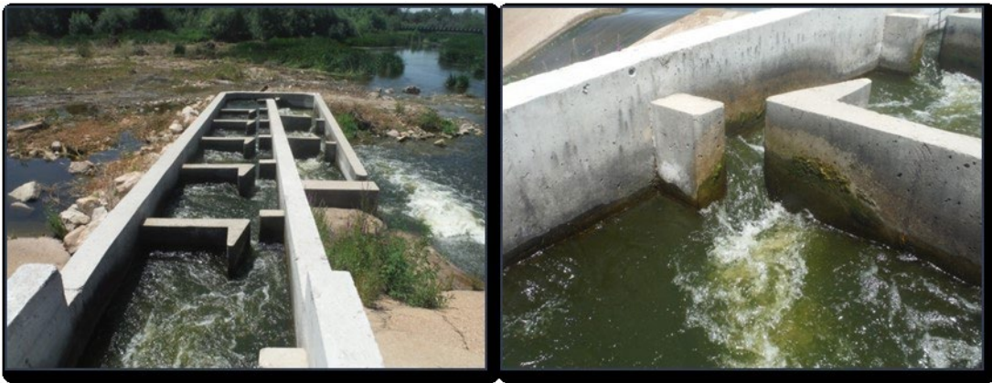
Figure 54. The inside of the fishway, and a detailed view of one of the vertical slots that connect two of the pools (right).
