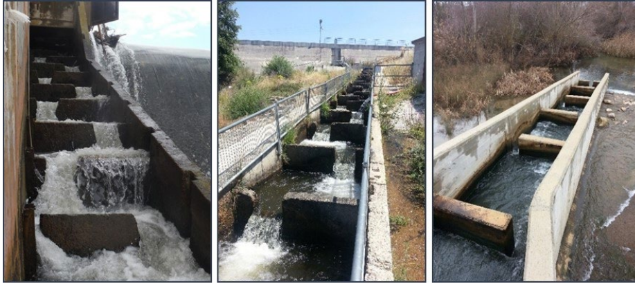
Figure 85. Fishways with different types of side protections: leeway too small (left), initially insufficient, although this was solved installing side protection fencing (centre) and leeway large enough (right).
