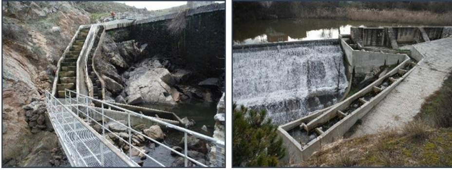
Figure 79. Footbridge (left) and concrete ramp (right) providing access to two fish passes.
