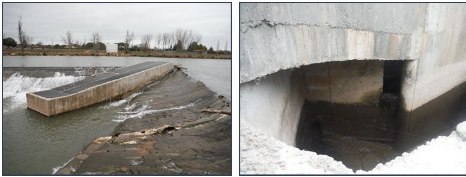
Figure 84. Examples of fish passes that are partially obscured by elements over them or excessive height of surrounding walls.
