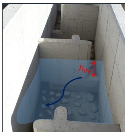
Figure 31. Example of the water depth (in red) as fish pass through a notch (the blue arrow shows the direction of the water flow).
