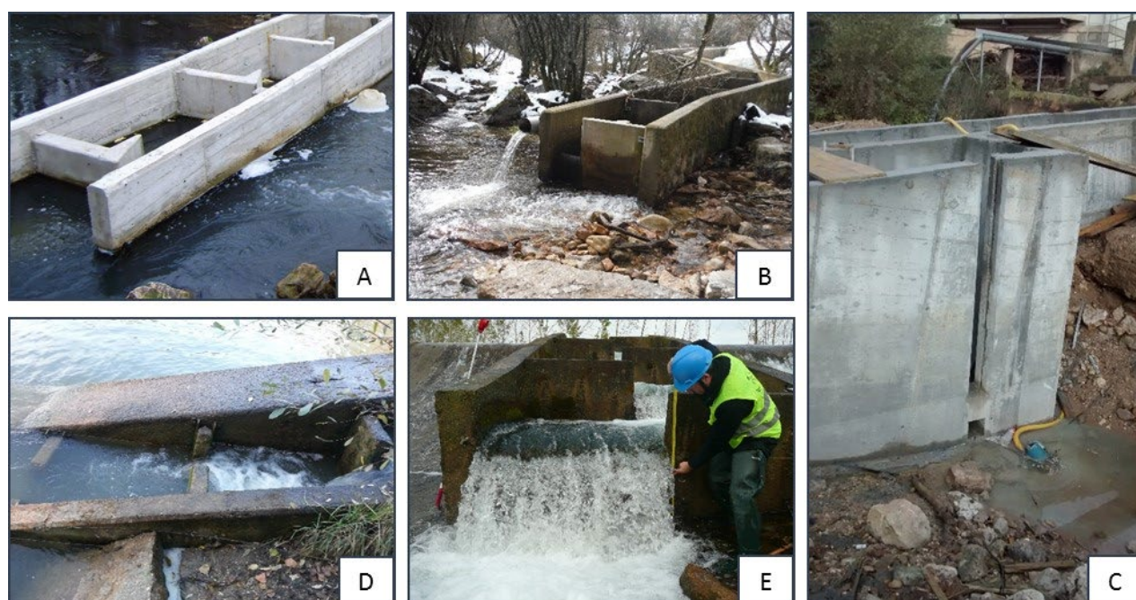
Figure 22. Different types of fishway entrances: vertical slot (A), surface notch + submerged orifice (B), submerged notch + submerged orifice (C), submerged notch (D), and surface notch (E).
