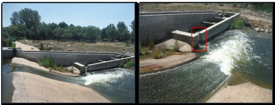
Figure 55. Water slide to attract fish (left) and its outflow next to the fishway entrance (in red) (right).
