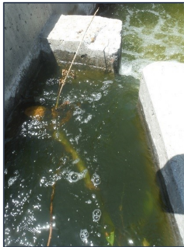
Figure 60. Partial obstruction observed in the slot connecting pools 3 and 4.
