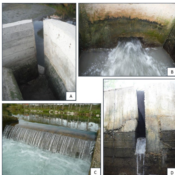
Figure 51. Most common types of exits: vertical slot (A), submerged orifice (B), surface notch (C) and submerged discharge (D).
