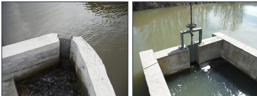
Figure 86. Different gates to regulate the water going into the fish pass.
