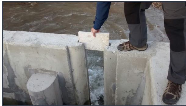
Figure 81. The sill height of a notch with a movable sill is modified to regulate the water level drop at the entrance.
